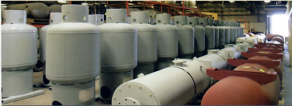
Shipping containers, filters, and air receivers
